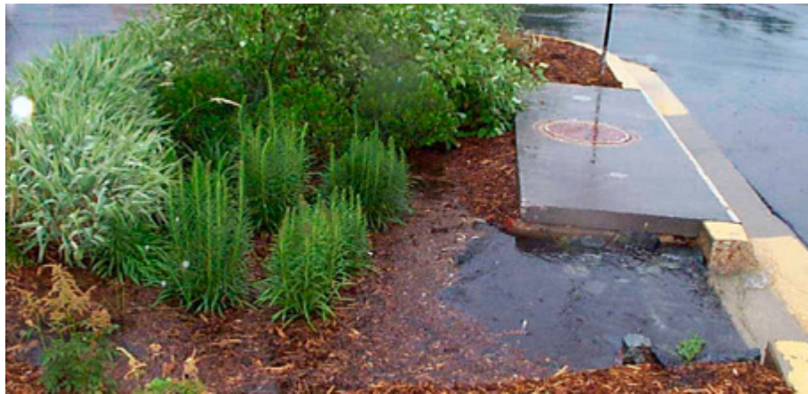
Curb inlet allows stormwater to enter planted median
