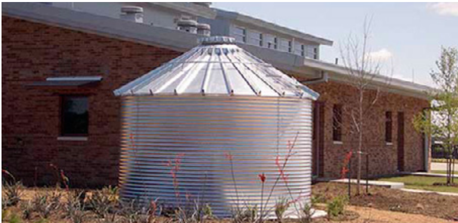
Cisterns as a center piece in a commercial district | Image Source: Climate Action Plans
