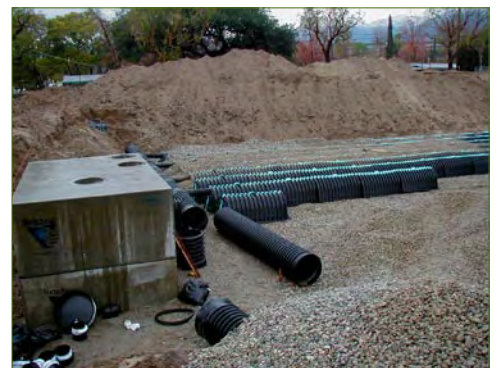
Two hundred and twenty infiltrator units below the ball field hold up to 95,200 gallons of water.
