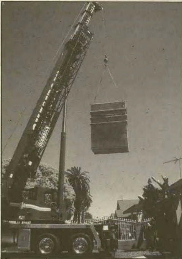
Each 1,800 gallon cistern unit was prefabricated off site and lifted over the house by a crane.
