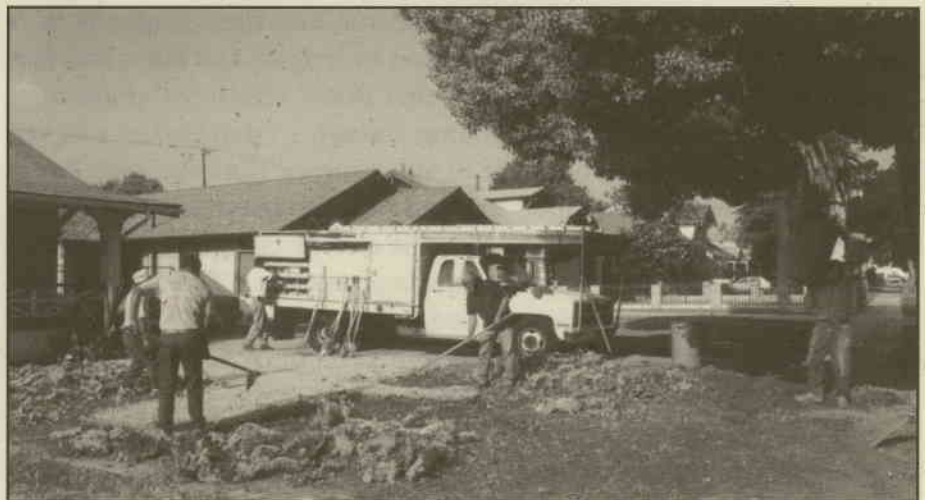
Most of the front yard was reconfigured to hold, rather than shed, rainwater.
