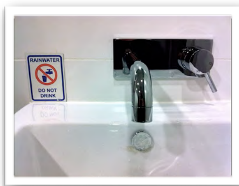
A faucet in the public restroom in Melbourne Water's brand-new building is served by captured rainwater.
