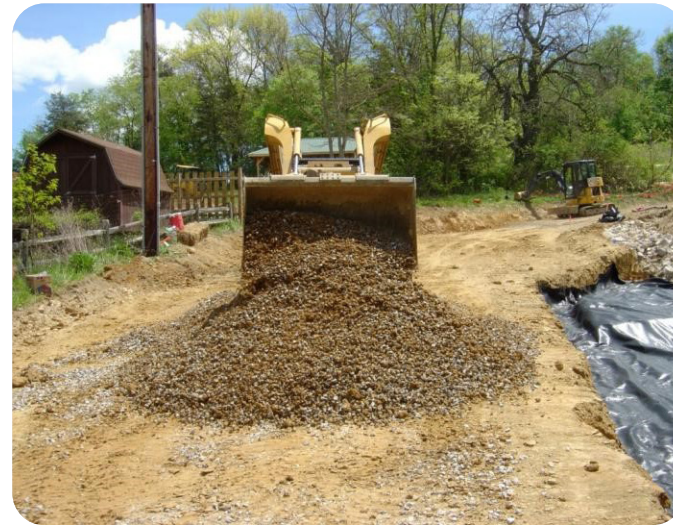
Figure 5. Mixing an engineered structural soil on site. The structural soil pictured here is composed of angular crushed stone that can support pavement and loose soil that can support root growth. (Photo: Susan Day)
